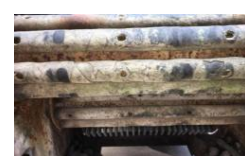
(b) Image of conveying roller
